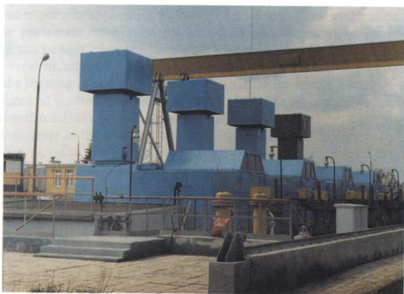
Fig. 5. Unit for partly closed enclosures (on openwork base) protecting the pumping engines in the Przepompownia Ropy ST-3 in Górk/Płocka.
